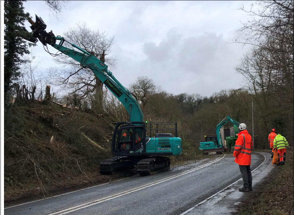
Figure 5. Tree Felling at Hendre FCC land. Note One Digger Felling and One Digger loading whole trees into a 24inch Chipper, woodchips fired into articulated lorry.
